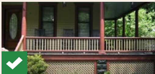
Historically Correct Handrail Height
