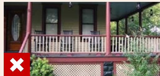
Handrail Height Too Tall
