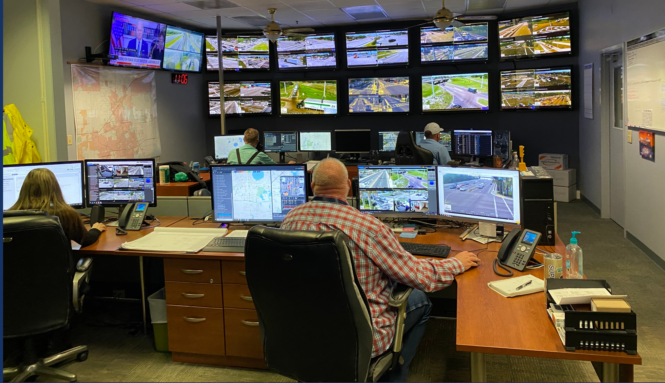
City of Lakeland Traffic Management Center
